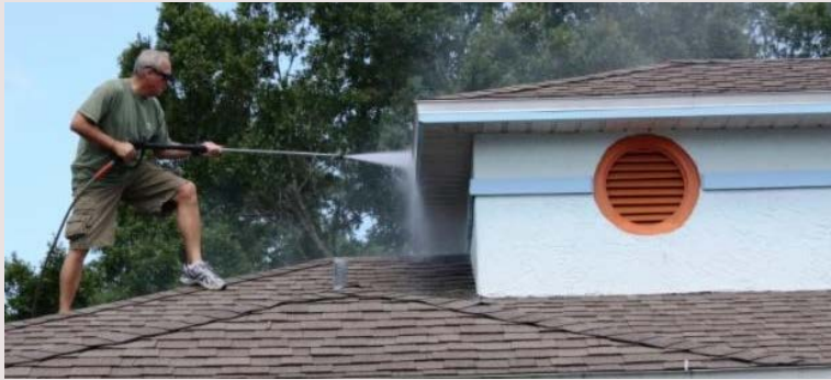
CFHLA Board Member and General Manager of the Sheraton Vistana Resort Glen Vlasic pressure washes the roof of a villa at Give Kids the World
